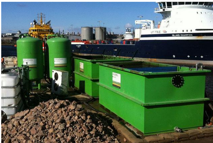
Soilutions_Pump and treat
